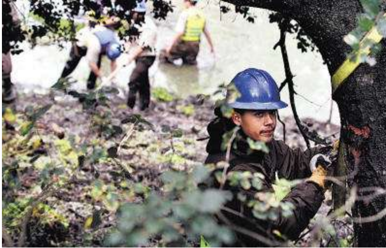
California Conservation Corp worker Michael Vera-Martinez attaches a winch to a tree to haul vegetation his crew removed from Pinto Lake on Monday (Shmuel Thaler/Sentinel)
